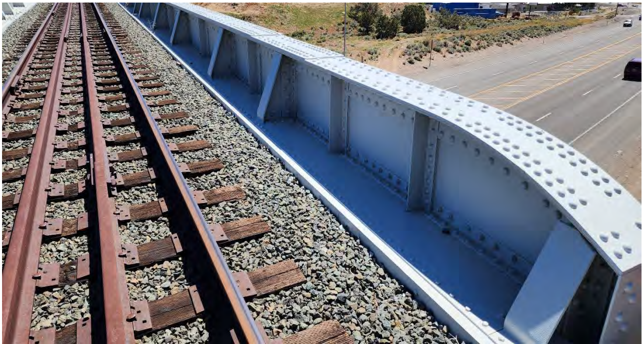
Knee Brace and Ballast Tub Plate on Left Side of Bridge @ North Span, Facing Southwest
