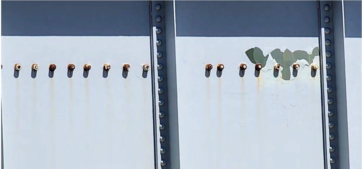
Main Girder At North span Facing East Rust forming and Paint Peeling on fasteners and panels
