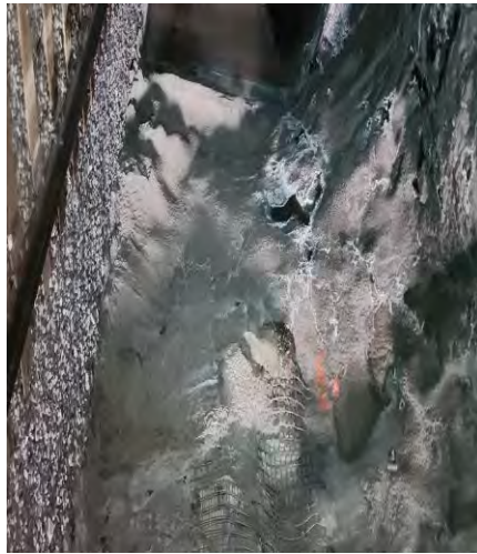
VCs Sta 858+70 additional seepage since previous inspection
