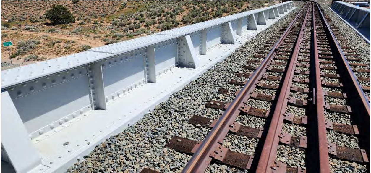
Main Girder and Ballast Tub Plate @ Left Side of Bridge Facing Northwest
