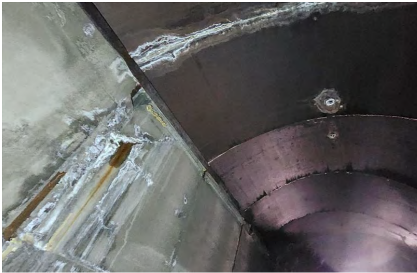
VCs Sta 858+16 Minor seepage
