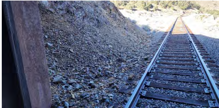
Clean ditch on left - large amount of soil and rock debris
